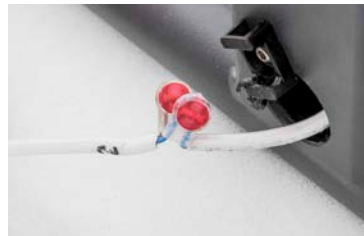
Connections outside of the frame
